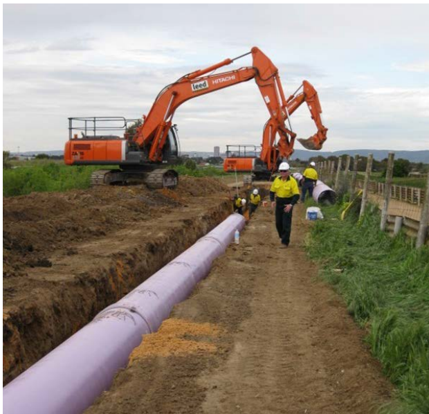
Figure 1: Purple pipe distribution network delivering recycled water to Australia's urban centres.
